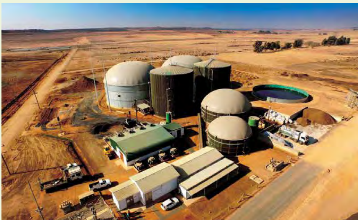
Bio2Watt biogas plant, Bronkhorstpruit
